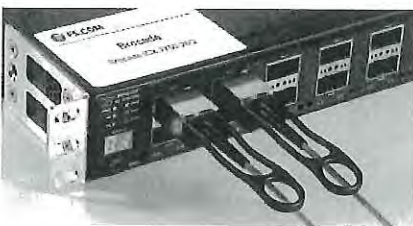
Brocade ICX 7750-26Q
